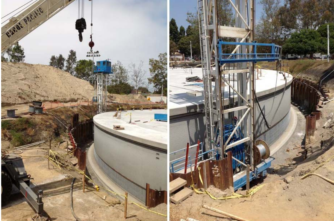
Penmar Water Quality Improvement Project - Concrete Tank Construction, Circumferential and Vertical Prestressing Operations
